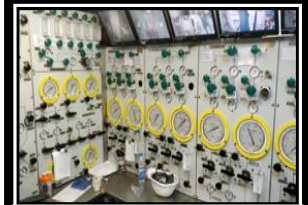
Saturation Dive Offshore Panel- Custom Make
